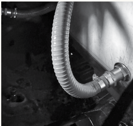
One of the many crucial DZR (Dezincification-Resistant) brass connections that allow the water to be safely drawn between environments with diverse materials and challenging access. ©David Cotterrell
